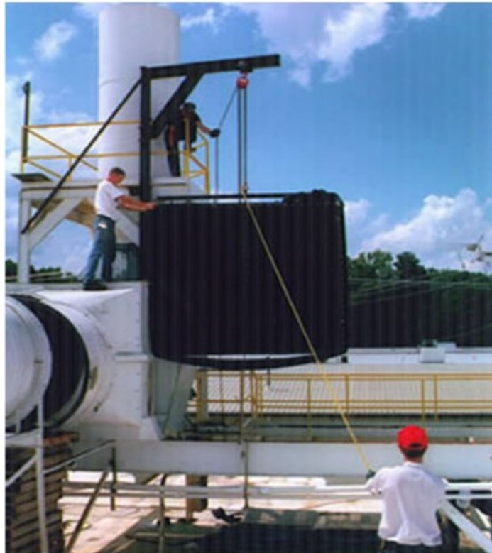
Field installation of Kimre tower packing, and mist eliminator cassettes. Top port entry facilitates ease of installation and maintenance. "On-line maintenance" permits replacement, or cleaning without process interruption.
